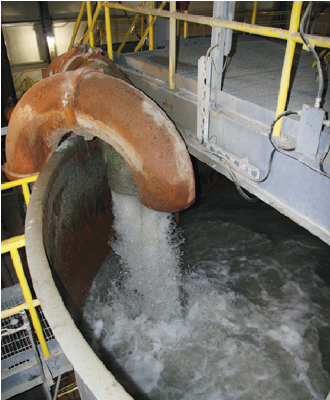
Photo above: Water from underground flows into the Water Treatment Plant
