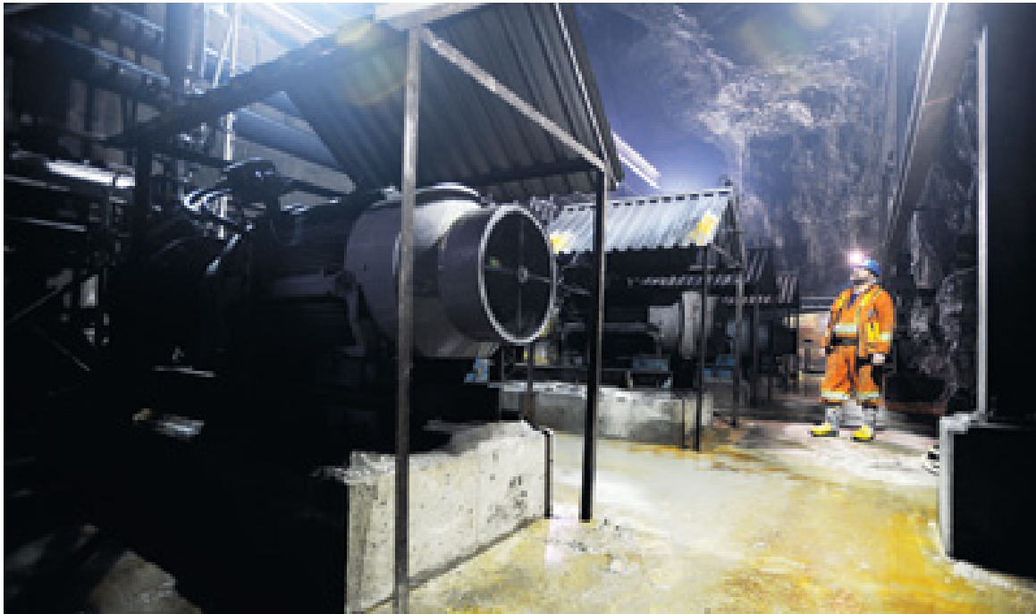
Photo above: The underground pumping station
