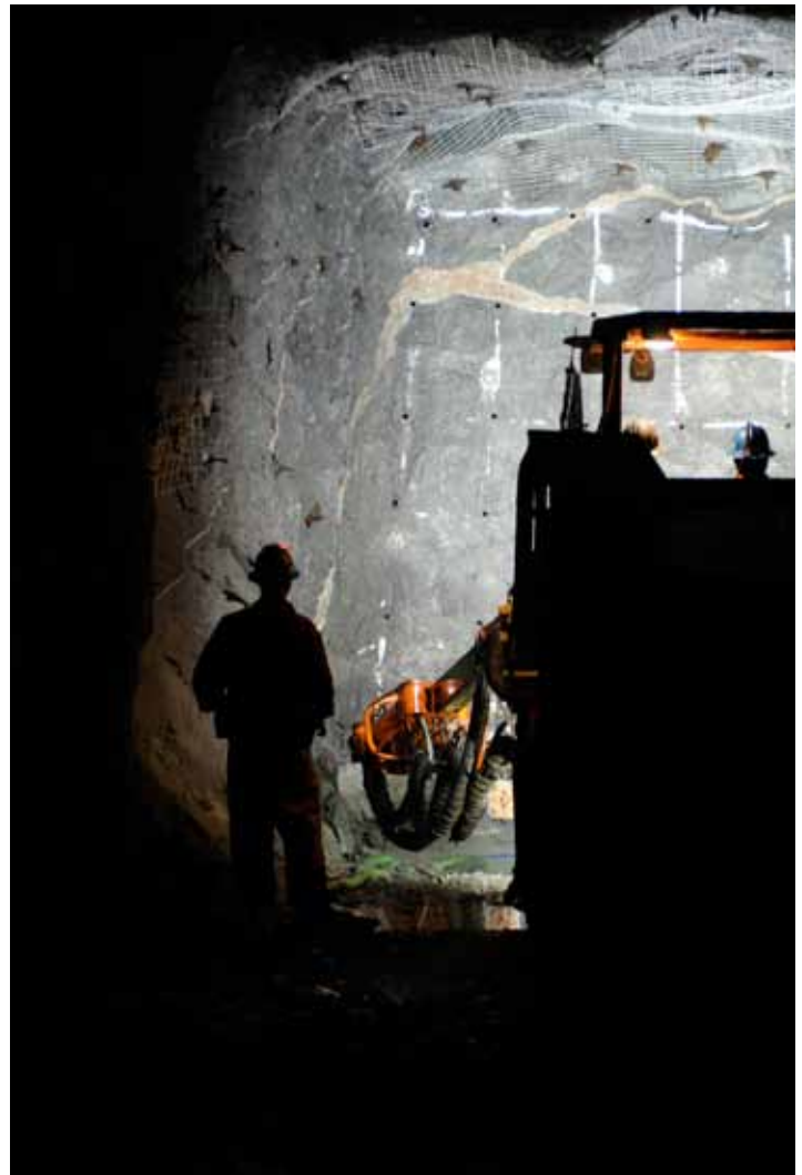
At Snap Lake Mine, a Jumbo drills holes in preparation for explosives.
