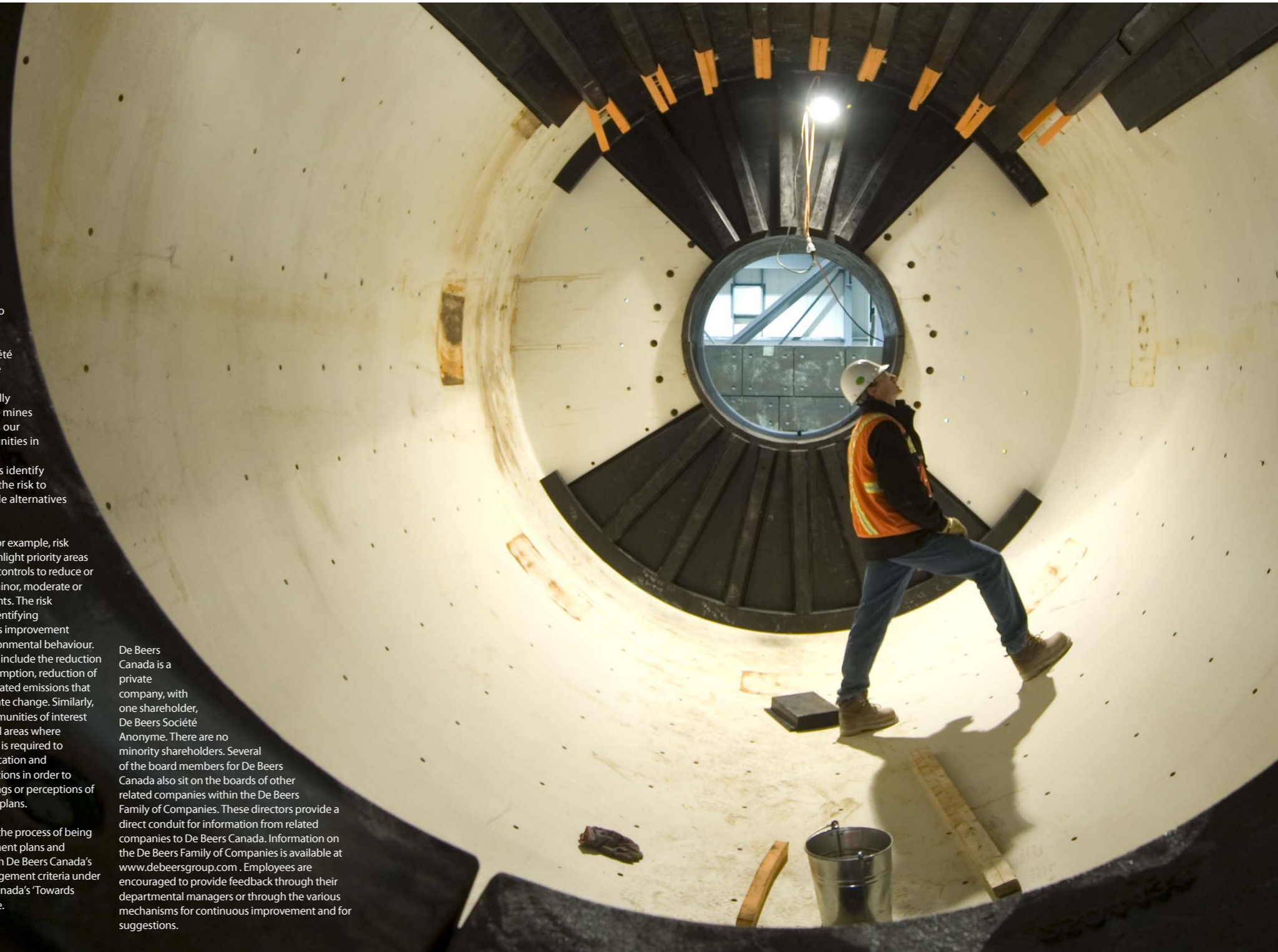
● The inside of the scrubber at Victor Mine is inspected before liner installation
